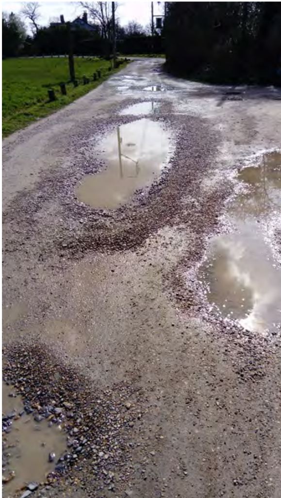
Figure 1 – Erosion on main through route
