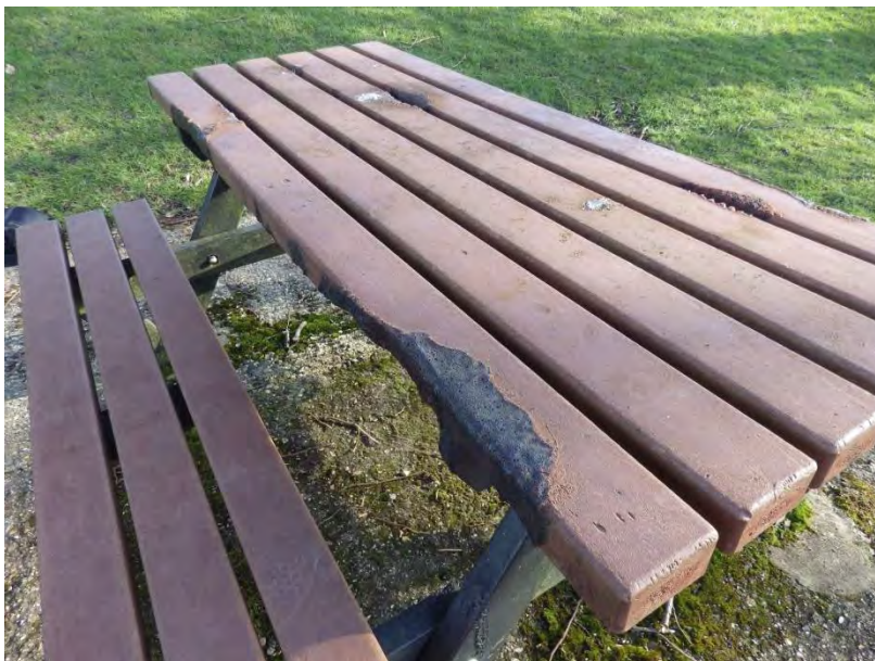
Fig. 1 – Burn damage to picnic table at Carvers Play Area
