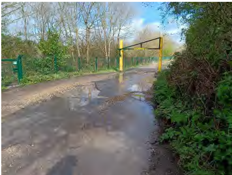
(Above) Existing pot holes at southern end of the track.
